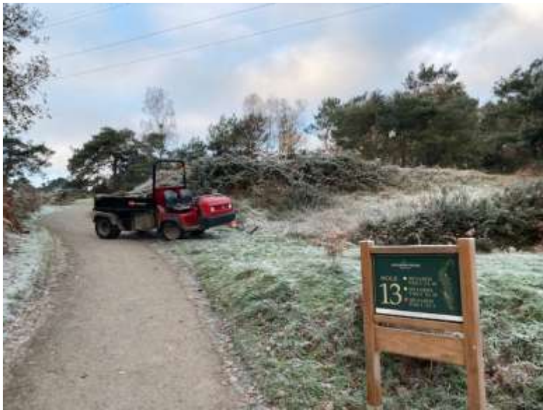
Some small clearance jobs around the course, like here at the front of the 13 th tee. Left shows before clearance
